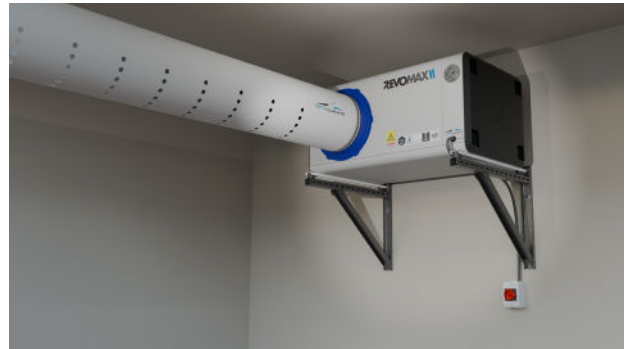
Wall mounted with air hose inside growing area
